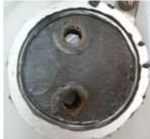
Fig. 9 Corroded Zinc coated iron plate
